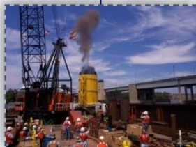
30 MN testing of 42mm dia. pipe pile, Woodrow Wilson Bridge, Washington, DC
