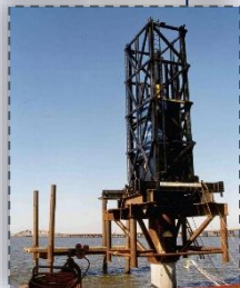
2200T Statnamic test on cylinder piles at St. George Island Bridge Applied Foundation Testing Inc.
