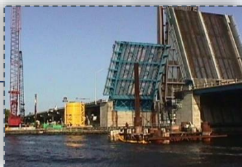
30MN load test 17th street Causeway Bridge Replacement in Ft. Lauderdale, Florida
